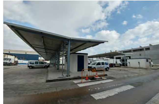
Smart electric vehicle recharging installation, FCC's fleet park in Barcelona.
